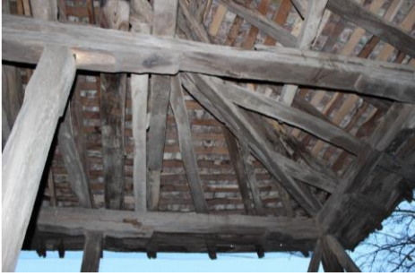
Deformation/ Deterioration Ordu Mosque
