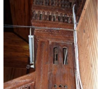
Plumbing system attachment Taşkıran Mosque
