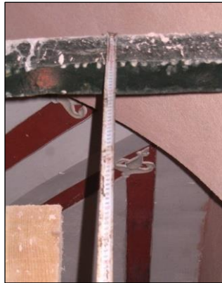
Figure 20. Tir rod inside the mosque (There are pounding marks on the tie rod and the width of the tie rod is 10 cm)
