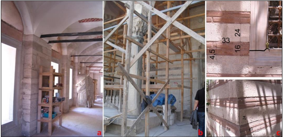
Figure 11. a-Cut stone material up to the level of the interior arch stirrup of the Zal Mahmud Pasha Mosque b-Qibla gate wall adjacent to the wall, jointed cut stone wall masonry c-Window profile detail and brick dimensions, stone dimensions
