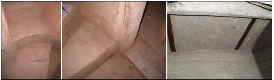
Figure 23. Step clamp on the left tribune ( mahfil ) staircase step leading to the tribune ( mahfil ) floor and tie rods on the staircase leading to the women's tribune (in a mosque) ( mahfil )
