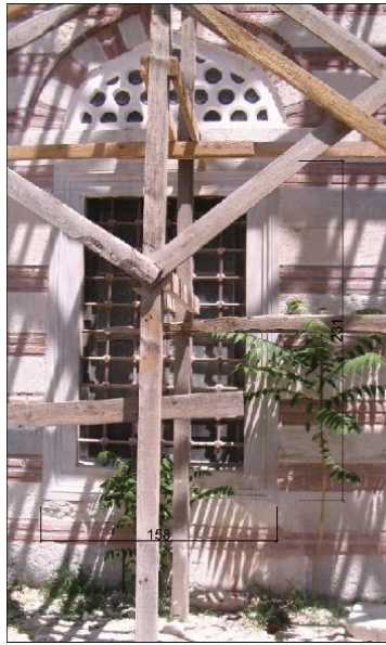
Figure 26. The 1st and 2nd-row windows of the mosque have a cover on the inside and knotted grille ( lokmalı parmaklık ) on the outside
