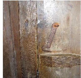
Corrosion effect Kondu Mosque
