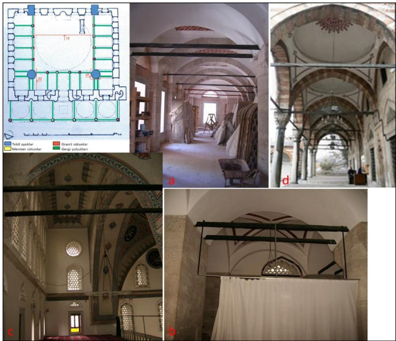
Figure 19. a-b-Harim floor single and double tie rods c-double tie rods of the women's cloister floor d-tie rods of the portico (of a mosque)
