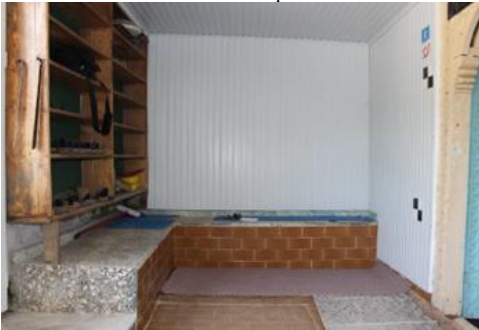
Use of unqualified materials Günebakan Mosque
