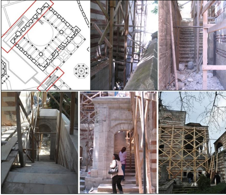
Figure 8. Stairs to the rear façade and photographs of the buttress; staircase from the lower madrasah to the upper madrasah
