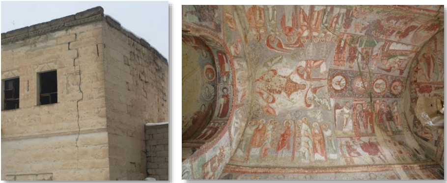
Figure 11. Crack in the facade wall
