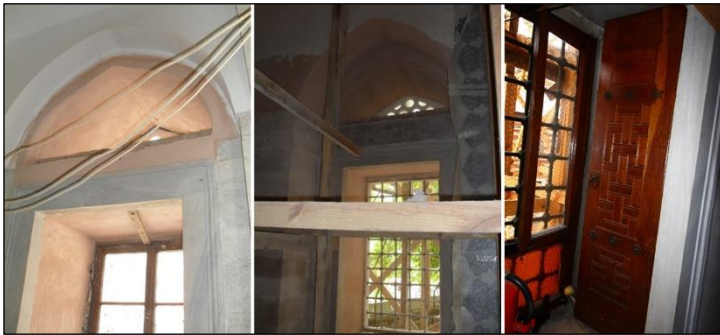
Figure 27. 1st and 2nd-row windows with inside cover and outside knotted grille iron railings
