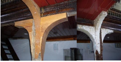
Use of unqualified materials Kondu Mosque
