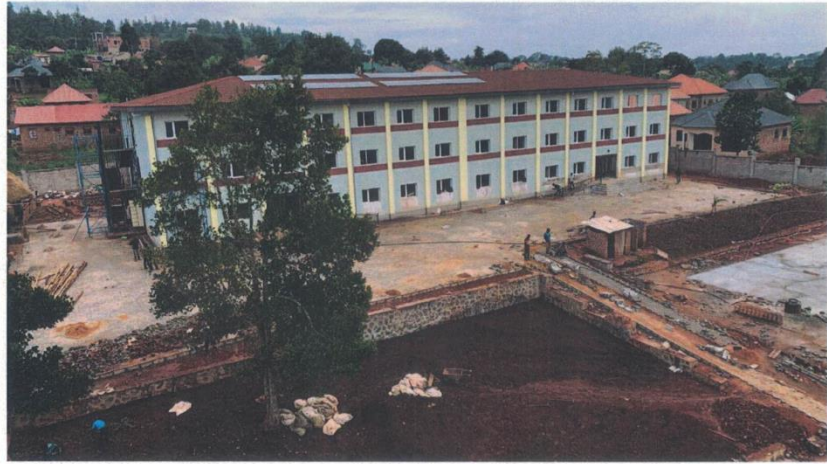
Construction of the educational complex in Nsagu 70% of work complete, wakiso district
