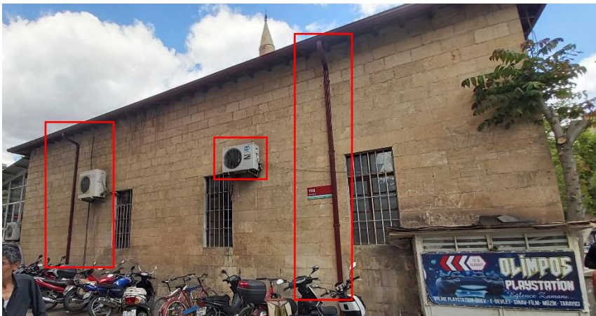
Figure 9. Air conditioning boxes and metal pipes on the wall of the mosque (Author's archive, 2022)
