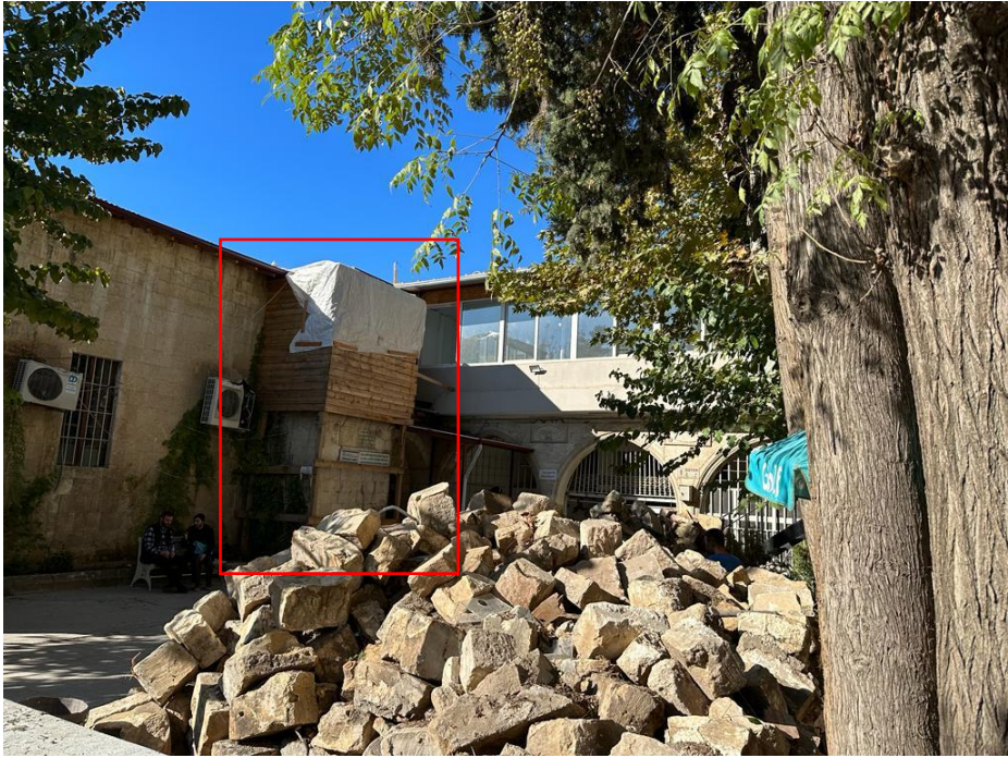
Figure 11. The minaret of the mosque after the earthquake (Author's archive, 2023)
