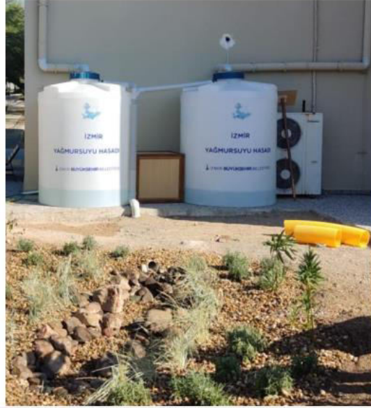
Figure 7. Two Rooftop Rainwater Storage Tanks and Connection to the Rain Garden
