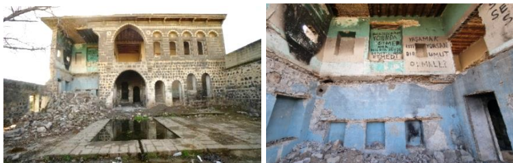
Figure 37. Wall and Floor Damage in the Ferit Mansion (2024)
