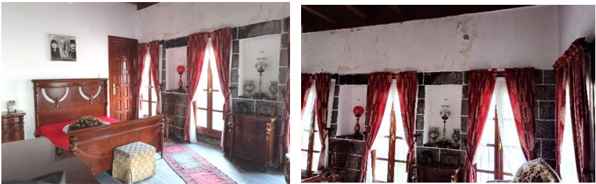
Figure 30. Gazi (Seman) Deterioration in Plaster Due to Moisture in the Mansion (2024)
