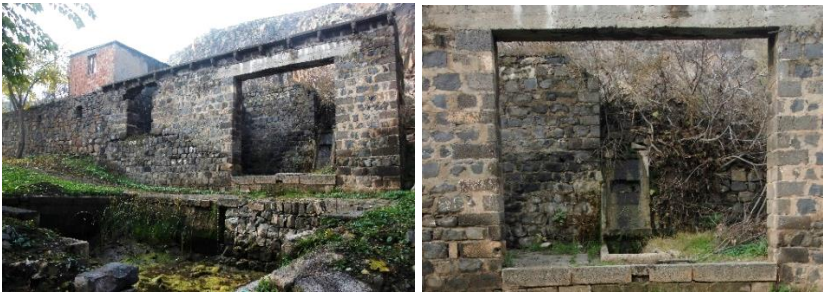
Figure 36. Ağuludere Mansion Floodplain and Collapsed Wall (2024)
