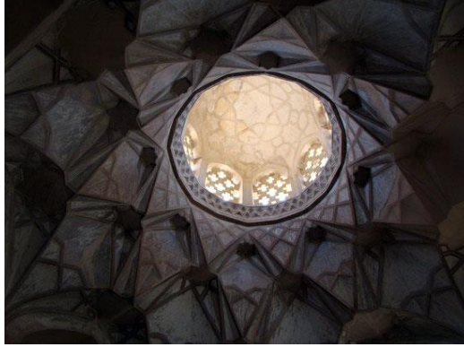
Figure 6. Haṣṭi's Natural Lighting System and Ceiling Cavity. Source: Iran Ministry of Culture and Islamic Guidance.
