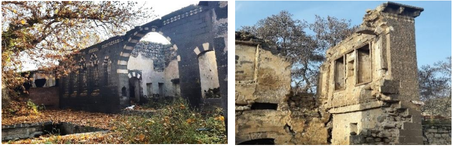
Figure 34. The Roof Cover and Collapsed Walls in the Ağuludere Mansion (2024)
