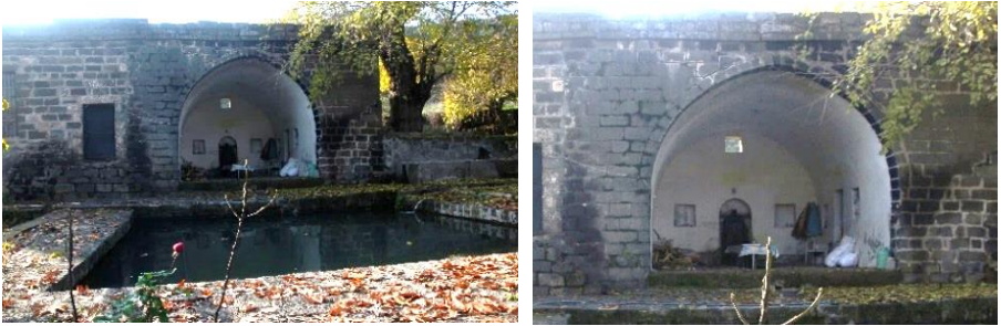
Figure 38. Moisture Damage in Bekir Pasha Mansion (2024)
