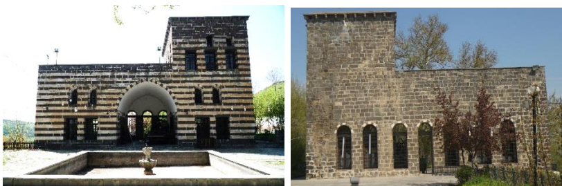
Figure 31. Partial Deterioration Due to Facade Contamination in Erdebil Mansion (2024)
