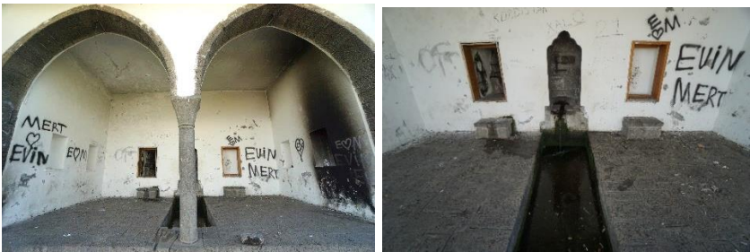
Figure 35. Deterioration Due to Neglect and Abandonment (2024)
