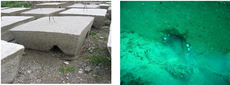
Figure 7. Construction of engineered octopus reefs (left) and their use by the octopus after deployment (right).
