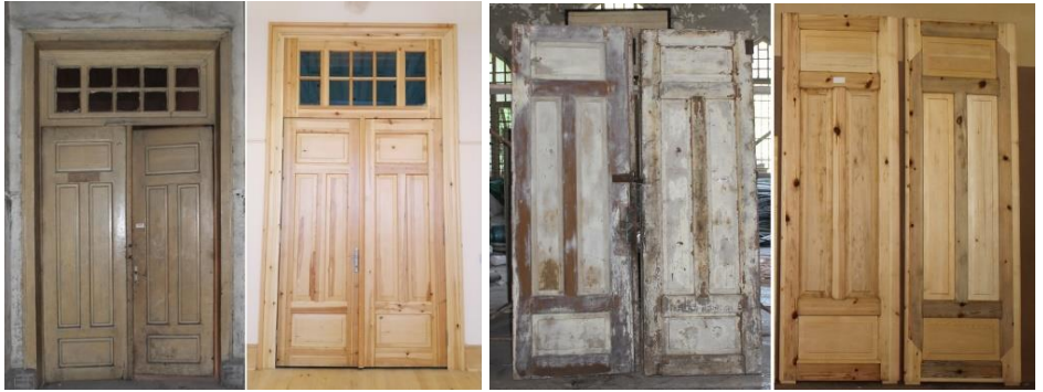
Figure 1041. The condition of the ground floor and first-floor doors before and after the application (Osmanoğlu, 2012-2017)
