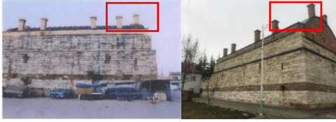
Concrete hats on the chimneys on the eastern facade of Rüstem Pasha Caravanserai before restoration (left) (restoration report, 2013) and brick hats after restoration (right)
