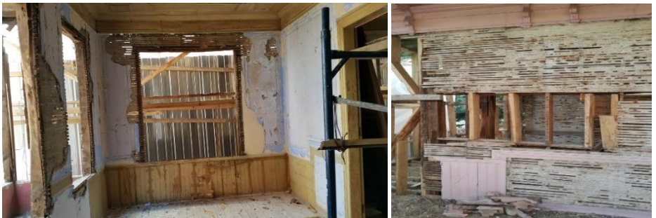
Figure 17. Interior Deteriorations (Osmanoğlu, 2017-2019)
