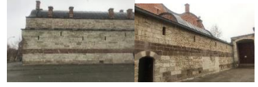
Rüstem Pasha Caravanserai after restoration from the west facade (left) and the upper cover view from the courtyard (right)
