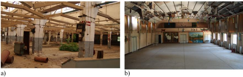
Figure 10. The idle condition of industrial heritage on the Sümerbank industrial campus in Nazilli.
