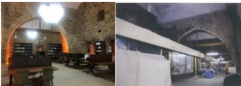
Shops attached to the stable part of the Rüstem Pasha caravanserai before restoration (left) and the stable part after restoration (right)
