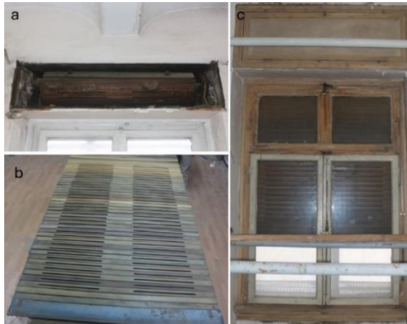
Figure 46. a) Interior of the shutter box, b) Example of the shutter during the repair process, c) Repaired shutter example installed on the window (Osmanoğlu, 2016-2024)
