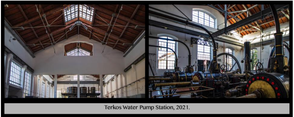
Figure 7. Terkos Water Pump Station (Photos: Author’s Archive, 2021).
