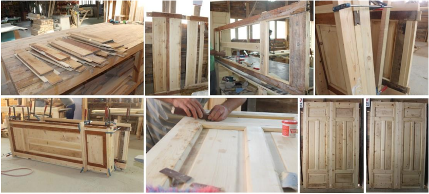
Figure 37. Disassembly of the doors and the integration of original components with newly manufactured elements using the consolidation technique (Osmanoğlu, 2012-2017)
