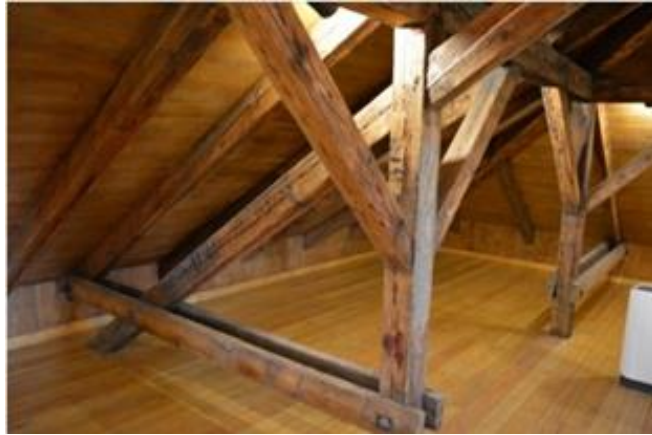
Figure 14. Original roof elements in the attic of the former German Embassy Building (Adalı, 2019)
