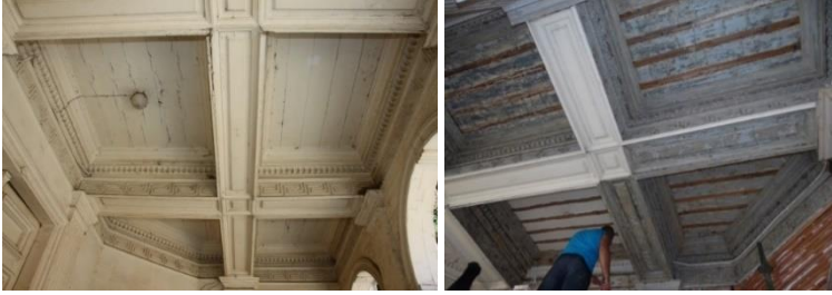
Figure 5. The condition of the building's balcony ceilings before restoration and the scraping applications (Osmanoğlu, 2015)
