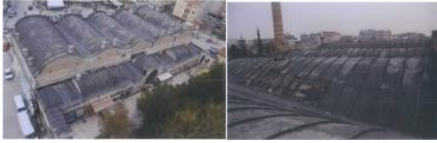
The upper cover of Rüstem Pasha Caravanserai before restoration (left and right)
