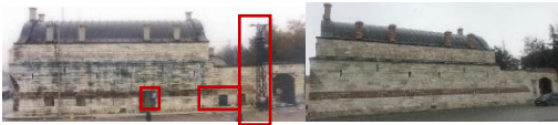
Additions to the west facade of the Rüstem Pasha Caravanserai before restoration, the color change and darkening of the material (left) and the west facade after restoration (right)
