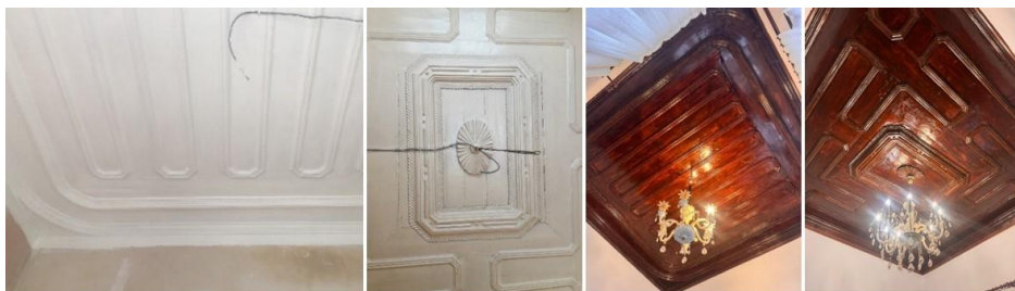
Figure 2. Wooden ceilings before restoration (Osmanoğlu, 2016) and after restoration (Osmanoğlu & Mukoviç, 2024)
