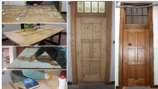
Figure 44. a) Cleaning application on the wooden door example using heat guns, b) cleaning with sandpaper, c, d) filling of gaps, e) the condition of the door after cleaning, and f) application of protective primer and varnish to the door (Osmanoğlu, 2016-2024).
