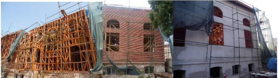
Figure 1. The restoration works included the renewal of the wooden frame system, lath strips, and plaster applications (Osmanoğlu, 2015).
