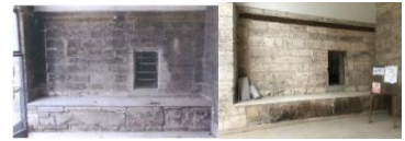
The bench at the entrance wall of the Rüstem Pasha Caravanserai before restoration (left) and the bench and flooring (right) at the entrance wall after restoration
