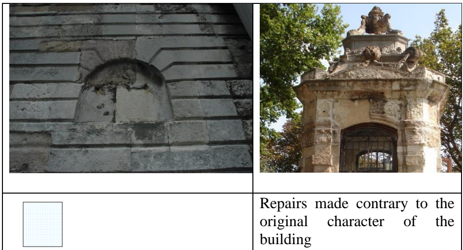
Figure 25. Mecidiye Gate Deterioration analysis (Author Archive, Bimtaş, 2009)
