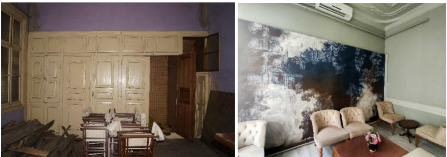
Figure 14. Before and after restoration of the original wooden cabinet (Osmanoğlu, 2016) and (Osmanoğlu & Mukoviç, 2024).
