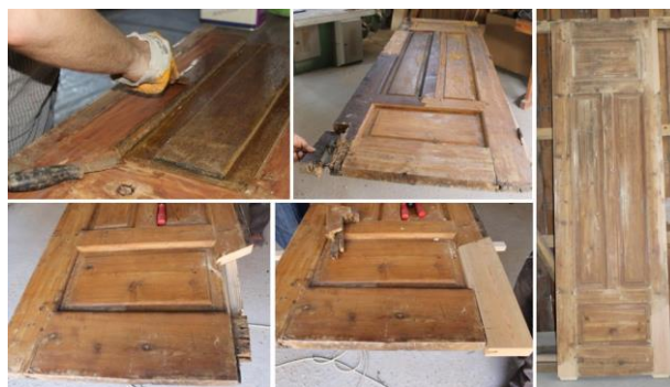
Figure 36. Details of the Consolidation Technique for Integrating Inferior Sections Following Chemical Cleaning (Osmanoğlu, 2012-2017)
