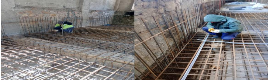
Figure 35. Anchoring of the piles and raft foundation reinforcements created to remain above the existing foundation, Restoration of the Building No. 5, Haydarpaşa Train Station, Istanbul, 2017-2024, (Osmanoğlu, 2017)
