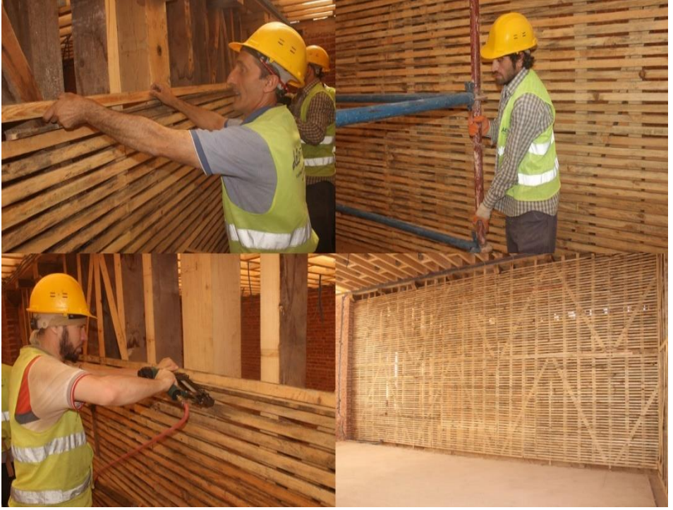
Figure 28. Repair of damaged and weakened wooden structural elements and lath, Restoration of Fatih Sultan Mehmet High School, Istanbul, 2010-2017, (Osmanoğlu, 2012)
