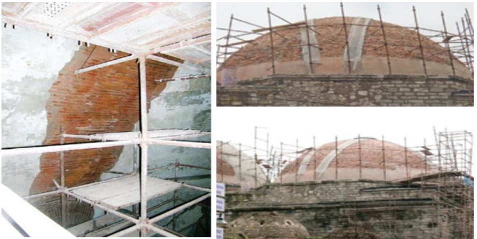
Figure 1. Repair of cracks in the right main dome of the Bayezid II Bath through stitching method, reinforcement application with carbon fiber tape in the left main dome, Restoration of the Bayezid II Bath, Istanbul, 2005-2014, (Osmanoğlu, 2008)
