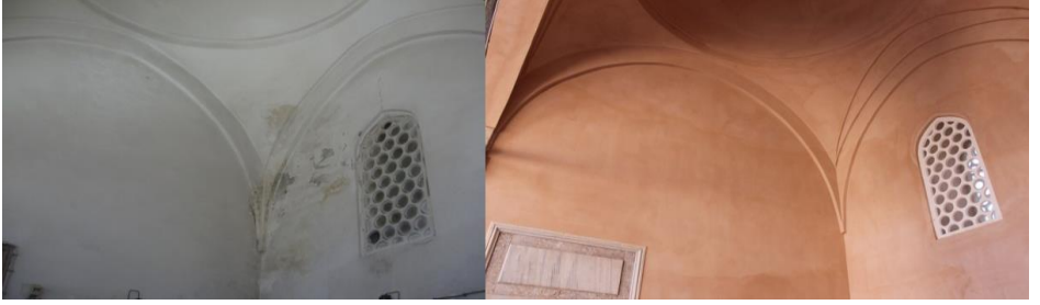
Figure 24. Repair of the iwan walls with the original mortar, rough plaster, and finish plaster as recommended in the material report, Restoration of Tabhane Building of Süleymaniye Complex, Istanbul, 2012-2018, (Osmanoğlu, 2015)
