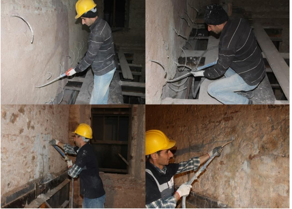
Figure 30. Hydraulic lime injection applications to cracks and voids in the walls, Restoration of Fatih Sultan Mehmet High School, Istanbul, 2010-2017, (Osmanoğlu, 2012)
