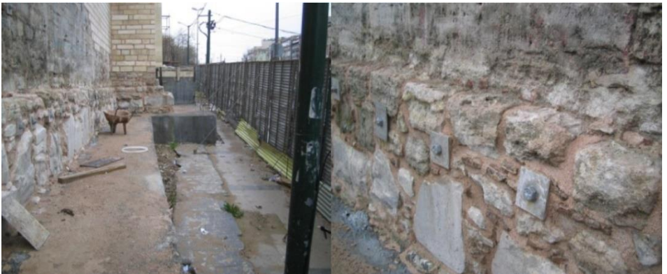
Figure 4. Anchorage application with connection bars on the inner and outer sides of the foundation walls on the south facade, Restoration of the Bayezid II Bath, Istanbul, 2005-2014, (Osmanoğlu, 2007)
