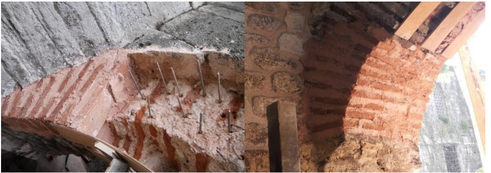
Figure 19. Removal of bricks that have lost their strength in the arches and application of anchorage with epoxy resin and steel rods for the installation of newly produced original bricks, Restoration of Tabhane Building of Süleymaniye Complex, Istanbul, 2012-2018, (Osmanoğlu, 2013)
