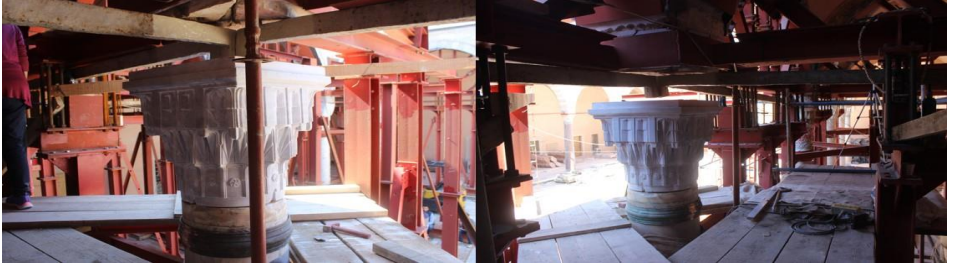
Figure 15. Installation of the repaired column capital, Restoration of Tabhane Building of Süleymaniye Complex, Istanbul, 2012-2018, (Osmanoğlu, 2014)
