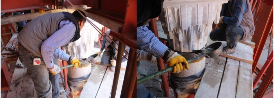
Figure 17. Application of pouring lead into the column rings (Restoration of Tabhane Building of Süleymaniye Complex, Istanbul, 2012-2018, (Osmanoğlu, 2014)
