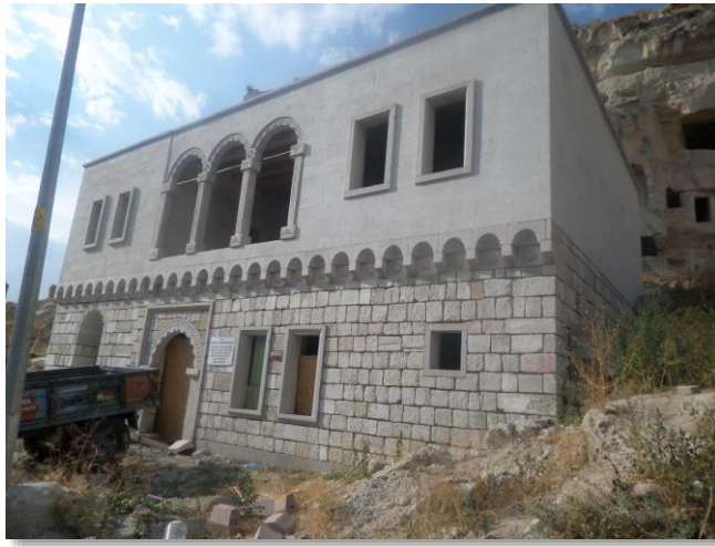
Figure 14. An example of a repair not in keeping with the local material (Aktaş, 2019)
