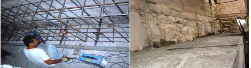
Figure 3. Reinforcement application using reinforced concrete for the foundations, Restoration of the Bayezid II Bath, Istanbul, 2005-2014, (Osmanoğlu, 2006)
