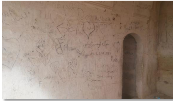
Figure 17. Vandalised walls in abandoned houses (Aktaş, 2019)
