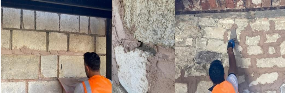
Figure 42. Consolidation of the masonry and joint mortars in the walls, the Restoration of Macedonia Tower, Edirne, 2024, (Osmanoğlu & Köse, 2024)
