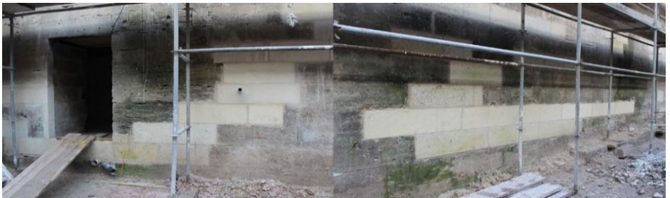
Figure 23. Repair of stone materials after the decay process, Restoration of Tabhane Building of Süleymaniye Complex, Istanbul, 2012-2018, (Osmanoğlu, 2012)
