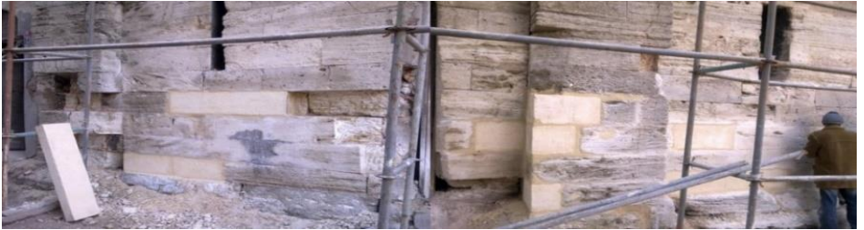
Figure 11. Stitching operation on stone walls, Restoration of Darüşşifa Building of Süleymaniye Complex, Istanbul, 2009-2016, (Osmanoğlu, 2010)
