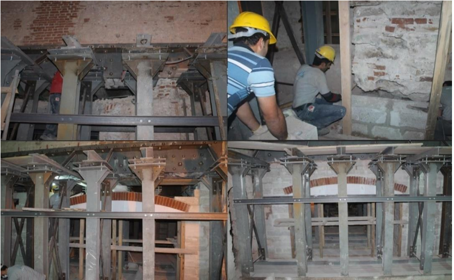
Figure 26. Suspension works of the basement supporting columns for repair procedures, Restoration of Fatih Sultan Mehmet High School, Istanbul, 2010-2017, (Osmanoğlu, 2010)
