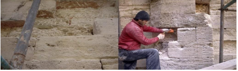
Figure 10. The process of removing deteriorated stone walls, Restoration of Darüşşifa Building of Süleymaniye Complex, Istanbul, 2009-2016, (Osmanoğlu, 2010)
