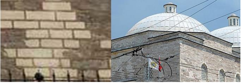
Figure 5. Stitching of the deterioration in the external facade wall masonry and consolidation application with binding mortar on the walls, Restoration of the Bayezid II Bath, Istanbul, 2005-2014, (Osmanoğlu, 2007)
