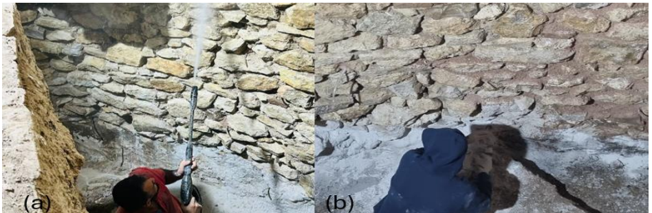
Figure 41. (a) Cleaning of the foundation walls with high-pressure water and (b) application of hydraulic lime injection to the walls, the Restoration of Macedonia Tower, Edirne, 2024, (Osmanoğlu & Köse, 2024)
