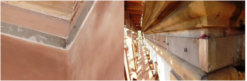
Figure 29. Application of stainless steel ties to strengthen the walls of the building, Restoration of Fatih Sultan Mehmet High School, Istanbul, 2010-2017, (Osmanoğlu, 2016)
