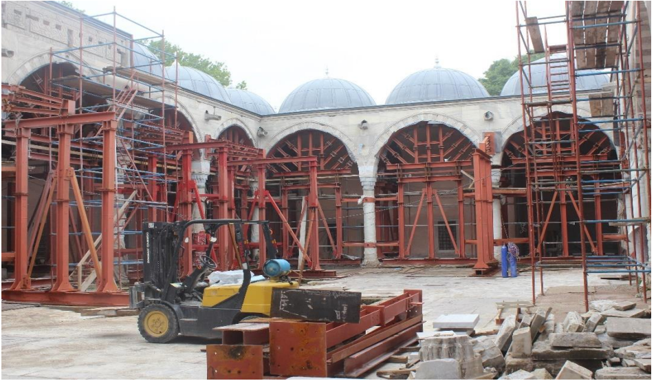
Figure 14. Application of suspension for the repair of the columns in the porticoes of the courtyard, Restoration of Tabhane Building of Süleymaniye Complex, Istanbul, 2012-2018, (Osmanoğlu, 2014)
