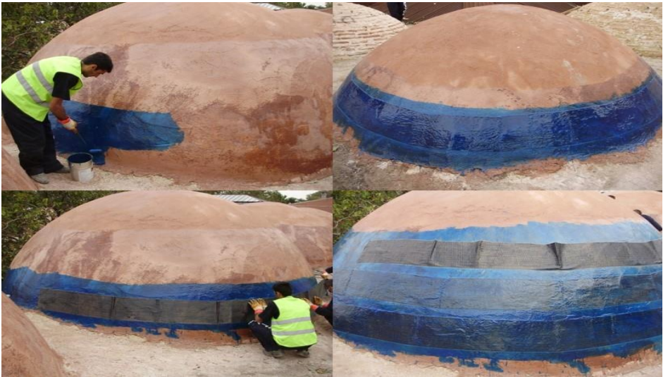
Figure 9. Reinforcement application using carbon fiber tape on the domes, Restoration of Darüşşifa Building of Süleymaniye Complex, Istanbul, 2009-2016, (Osmanoğlu, 2012)
