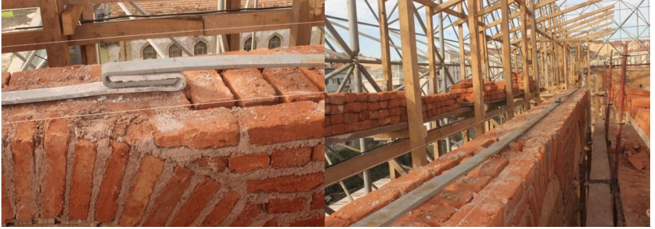
Figure 32. Reinforcement along the length of the wall beneath the supporting steel beams of the arch ceiling, Restoration of Fatih Sultan Mehmet High School, Istanbul, 2010-2017, (Osmanoğlu, 2015)
