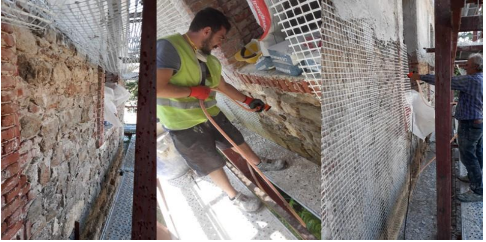
Figure 45. Application of plaster reinforcement with glass fiber mesh, the Restoration of Reji Buildings, Edirne, 2017-2018, (Osmanoğlu, 2018)
