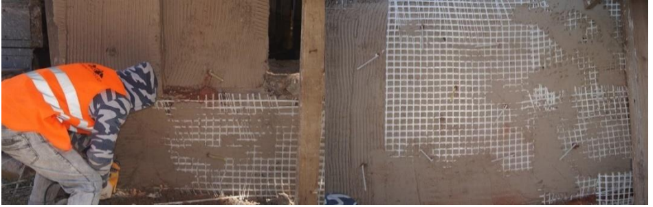
Figure 38. Strengthening works for walls and plasters using glass fiber-based reinforcement mesh, Restoration of the Building No. 5, Haydarpaşa Train Station, Istanbul, 2017-2024, (Osmanoğlu, 2020)
