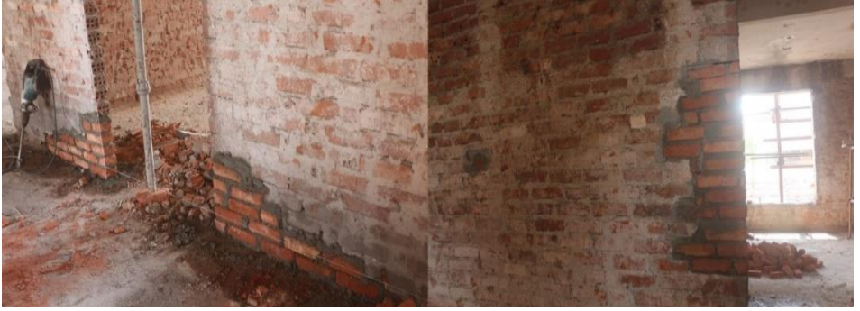
Figure 37. Stitching applications using original materials and techniques to repair cracks and material deterioration in the walls, Restoration of the Building No. 5, Haydarpaşa Train Station, Istanbul, 2017-2024, (Osmanoğlu, 2018)
