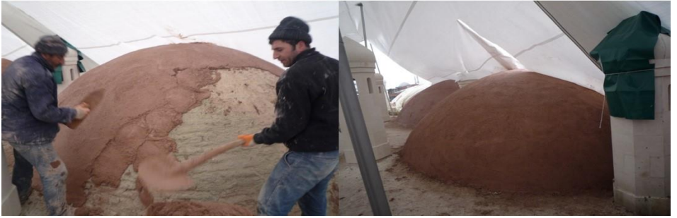
Figure 7. Consolidation application with original plaster after injection and stitching work on the domes, Restoration of Darüşşifa Building of Süleymaniye Complex, Istanbul, 2009-2016, (Osmanoğlu, 2012)
