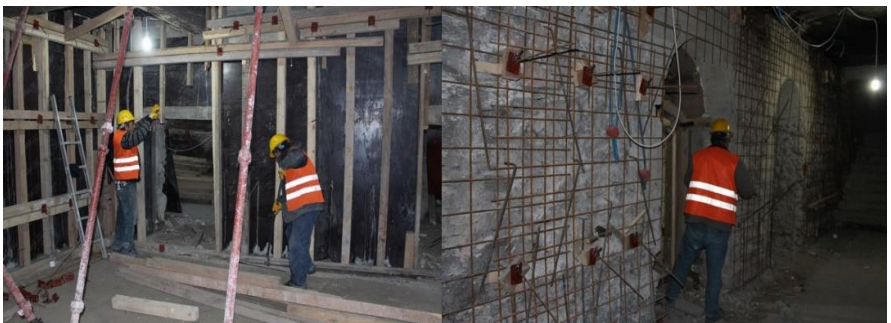
Figure 40. Application of sprayed concrete onto the steel mesh reinforcements anchored to the existing load-bearing walls, the Restoration of Akşemsettin Primary School, Istanbul, 2013-2016, (Osmanoğlu, 2013)
