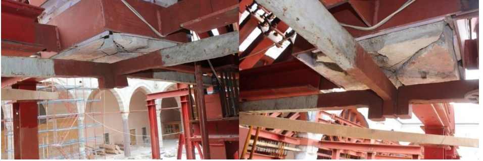
Figure 18. Cleaning and painting the ties with anti-rust paint, Restoration of Tabhane Building of Süleymaniye Complex, Istanbul, 2012-2018, (Osmanoğlu, 2014)
