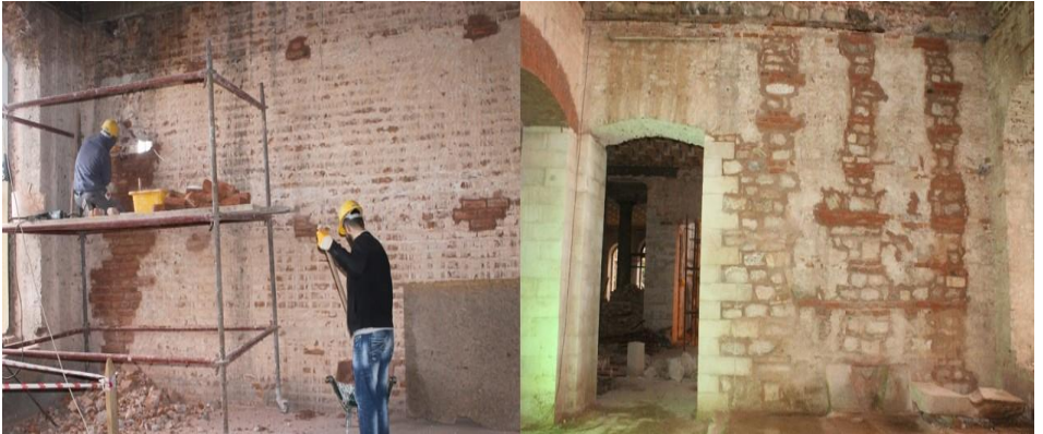
Figure 31. Removal of damaged and unusable bricks due to structural damage and stitching applications made with original forms, materials, and techniques, Restoration of Fatih Sultan Mehmet High School, Istanbul, 2010-2017, (Osmanoğlu, 2012)
