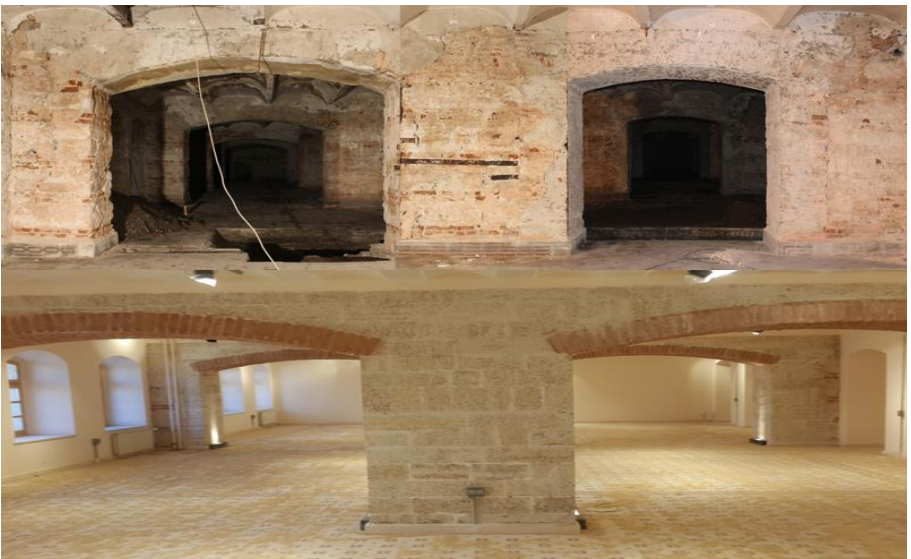
Figure 27. Before and after conditions of consolidation and reinforcement works on the basement columns, Restoration of Fatih Sultan Mehmet High School, Istanbul, 2010-2017, (Osmanoğlu, 2010-2017)
