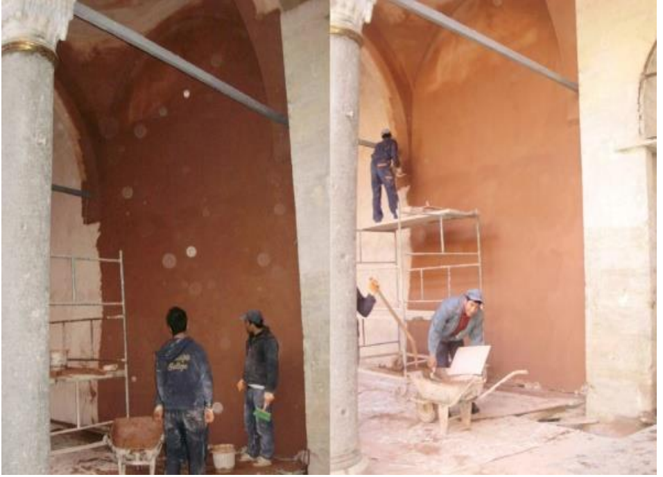
Figure 13. Application of original rough plaster and finish plaster on plastered wall surfaces. Restoration of the Süleymaniye Complex Darüşşifa, Istanbul, 2009-2016, (Osmanoğlu, 2013)
