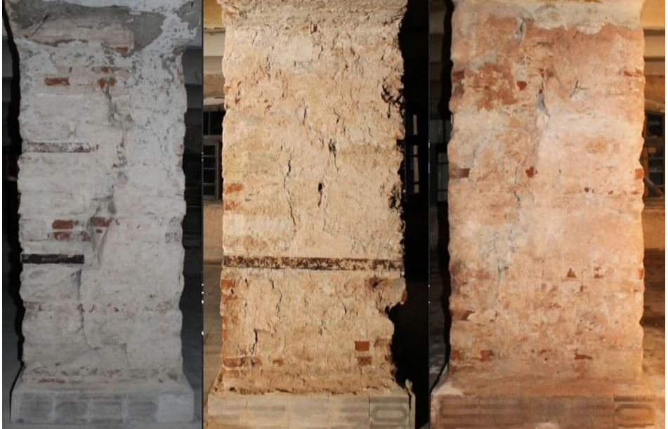
Figure 25. Damage assessment studies on the supporting columns in the basement, Restoration of Fatih Sultan Mehmet High School, Istanbul, 2010-2017, (Osmanoğlu, 2010)
