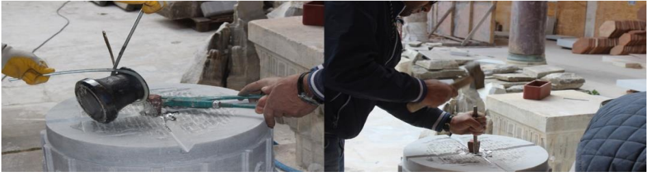
Figure 16. Placement of the keys on the column capital and pouring of lead into the key socket, Restoration of Tabhane Building of Süleymaniye Complex, Istanbul, 2012-2018, (Osmanoğlu, 2014)
