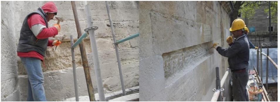
Figure 22. Removal of damaged material from the stone walls using the decay method, Restoration of Tabhane Building of Süleymaniye Complex, Istanbul, 2012-2018, (Osmanoğlu, 2012)
