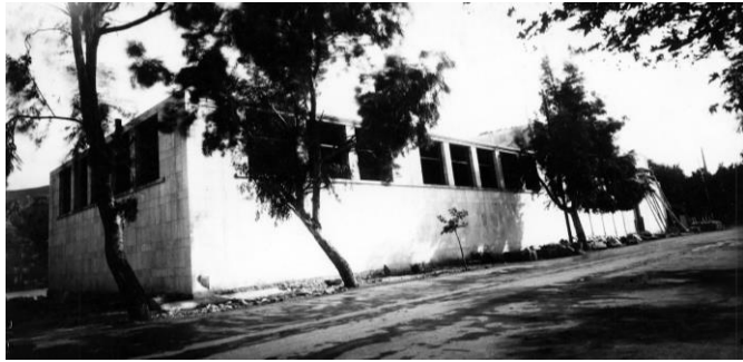
Figure 18. A general view of the construction process. (MIT Aga Khan Documentation Center, Michel Ecohard Archives, 1935)
