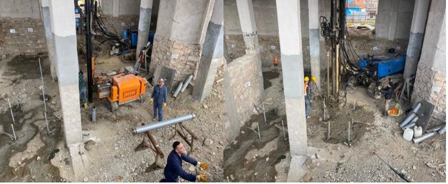
Figure 34. Strengthening the building foundation through micro-pile applications, Restoration of the Building No. 5, Haydarpaşa Train Station, Istanbul, 2017-2024, (Osmanoğlu, 2017)
