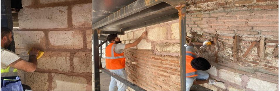
Figure 43. Consolidation applications in joint mortars, the Restoration of Macedonia Tower, Edirne, 2024, (Osmanoğlu & Köse, 2024)
