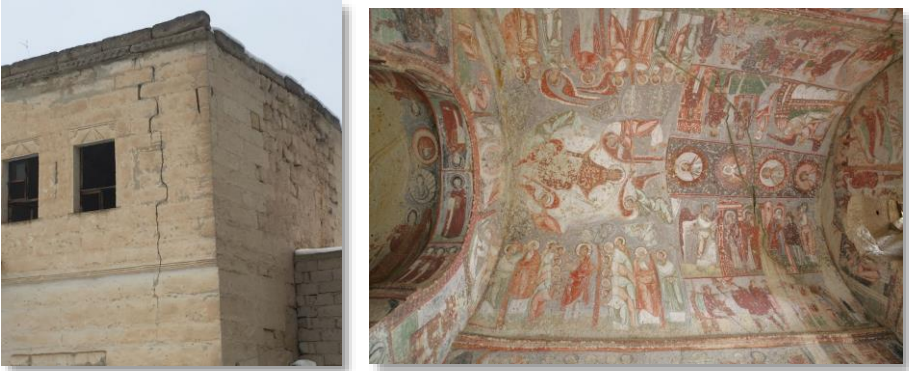
Figure 11. Crack in the facade wall, Figure 12. Crack in the vault of Çavuşin Church (Aktaş, 2019)
