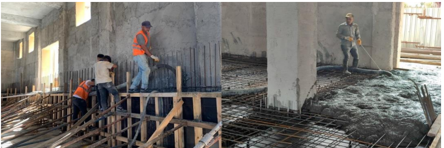
Figure 36. Pouring concrete into the raft foundation reinforcements constructed to strengthen the existing foundation, Restoration of the Building No. 5, Haydarpaşa Train Station, Istanbul, 2017-2024, (Osmanoğlu, 2017)
