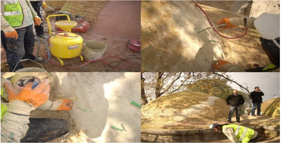
Figure 8. Stages of hydraulic lime injection application for dome cracks, Restoration of Darüşşifa Building of Süleymaniye Complex, Istanbul, 2009-2016, (Osmanoğlu, 2012)
