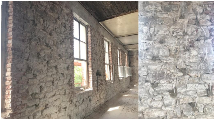
Figure 44. Consolidation of the perimeter walls through injection, the Restoration of Reji Buildings, Edirne, 2017-2018, (Osmanoğlu, 2017)
