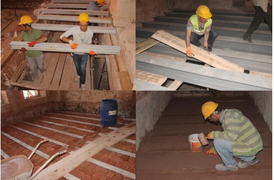
Figure 33. Reinforcement and consolidation applications on arch ceilings with reduced load-bearing capacity due to section loss in iron profiles and damage to the bricks forming the arch, Restoration of Fatih Sultan Mehmet High School, Istanbul, 2010-2017, (Osmanoğlu, 2016)
