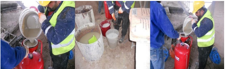
Figure 20. Preparation for hydraulic lime injection, Restoration of Tabhane Building of Süleymaniye Complex, Istanbul, 2012-2018, (Osmanoğlu, 2013)
