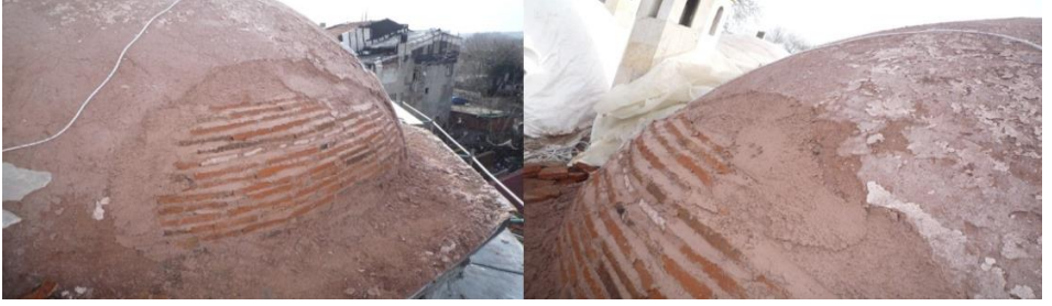
Figure 6. Stitching applied with bricks produced in original form, technique, and content on the domes, Restoration of Darüşşifa Building of Süleymaniye Complex, Istanbul, 2009-2016, (Osmanoğlu, 2012)
