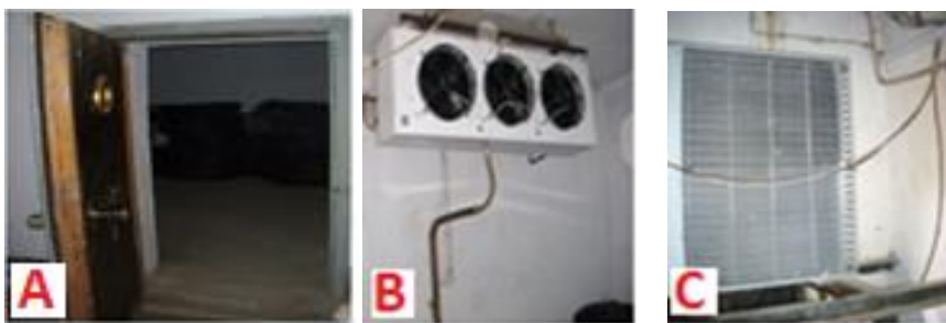
Figure 1. Cold store (A), evaporator (B), condenser (C)
